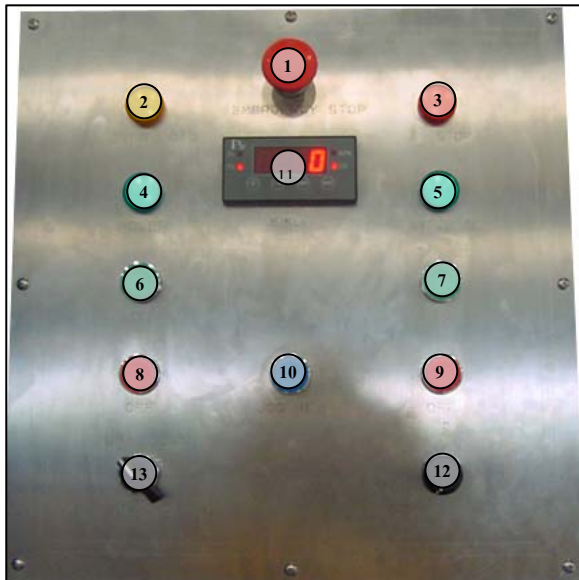
Left Control Panel
