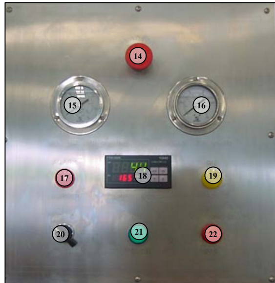
Right Control Panel
